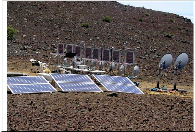
Figure 8-2 Solar Powered WPT Equipment in Hawaii (May 2008)
