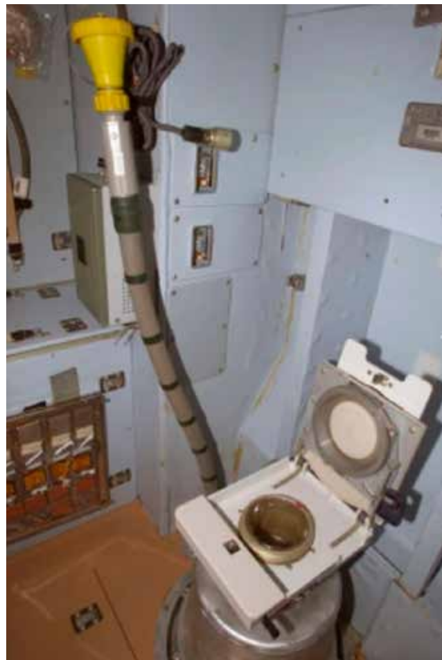
The urine reclamation system in the ISS toilet is one of the systems most prone to breakdown.
